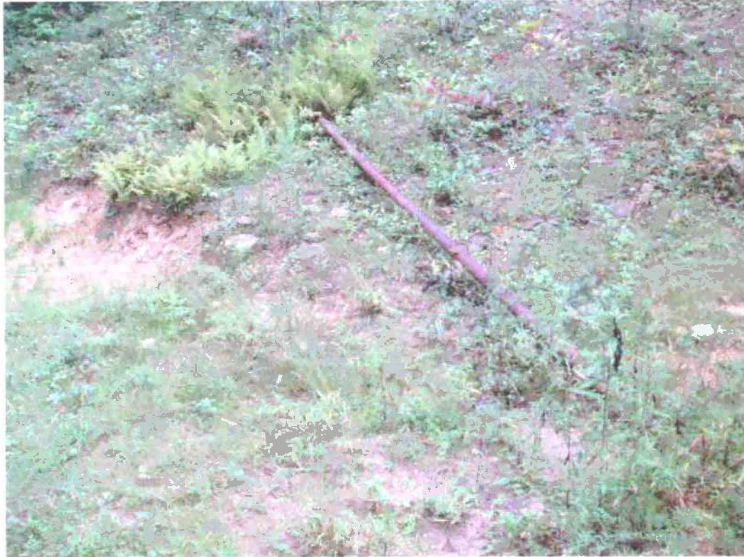
Figure 4. Rusted metal gas line exposed by erosion in slope adjacent to third Keyspan gas well visited, located approximately 2,600 feet Due North of the first well. Gas line trends from well to monitoring station approximately 200 feet southeast, and then continues underground to tie in with line that connects first two wells visited (compare to Figures 1 and 2).
